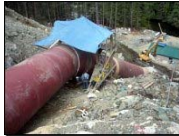
Penstock into the Power House
