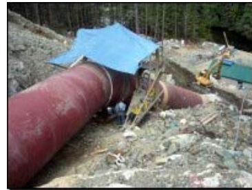
Penstock into the Power House
